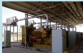
Chad 4MW diesel power plant
