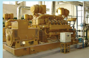
Series 127 gas generator set
