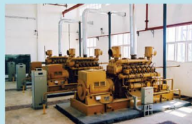
Natural gas power plant of W-EGTP
