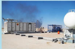
Power plant of Iraq Rumaila oil field
