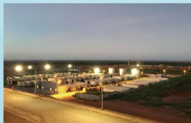
Tanzania 60MW diesel power plant
