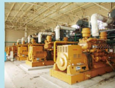
Henan Shuanghui biogas power plant
