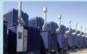
Saudi Arabia 75MW diesel power plant
