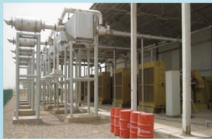
Chad generator set project
