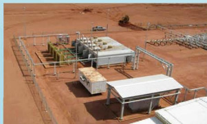
Associated gas power plant in Sudan
